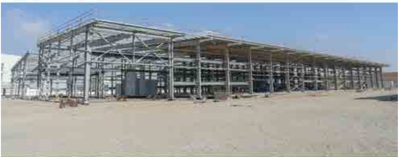
Client : M/S. AMANA CONTRACTING AND STEEL BUILDING CO. WLL Project : ACE BASE EXPANSION FOR M/S. SCHLUMBERGER
