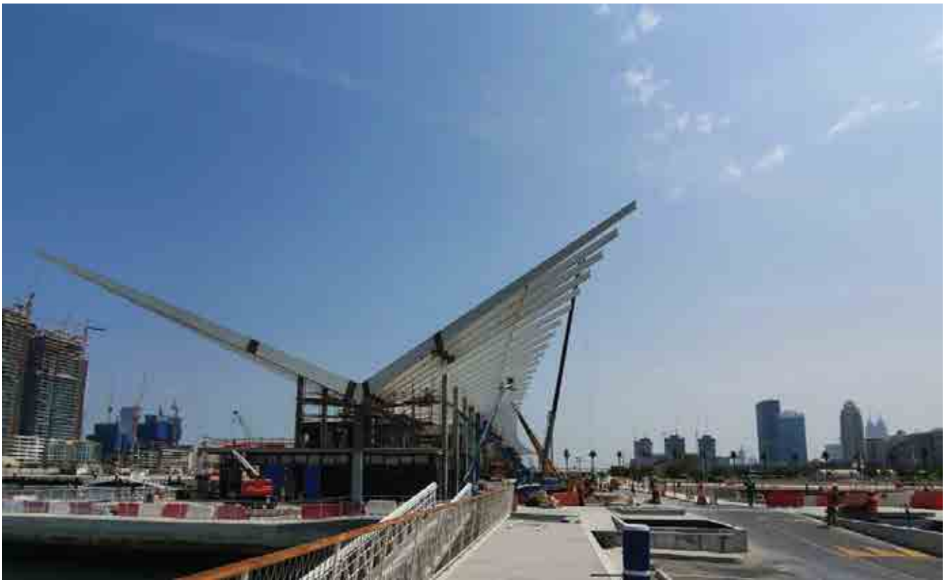
Client : M/S. AMANA STEEL BUILDINGS CONTRACTING LLC Project : DUBAI HARBOUR MASTERS BUILDING
